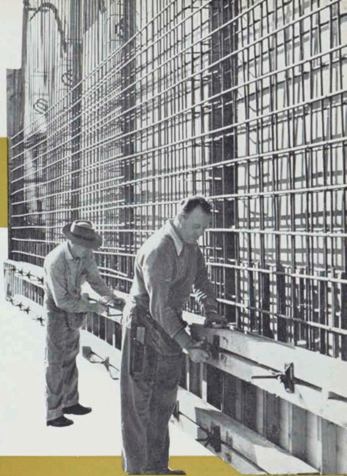
Gladstone Road Overbridge, Mount Albert, Auckland. Securing the boxing prior to the pouring of concrete are Norm. Harmsworth, at rear, and Dave Phillips. Engineers: Harrison & Grierson & Partners; Contract Manager: Bob Foster; Foreman: Tom Edmunds.
