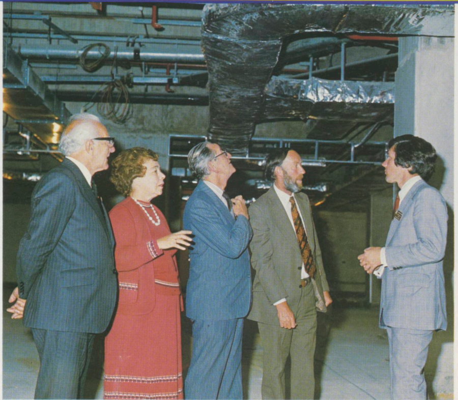
The directors of Fletcher Holdings recently paid a visit to the Dunedin Hospital ward block construction site, accompanied by the Hospital Board chairman, Mrs Dorothy Fraser. In this photograph are, from left, Sir John Marshall, Mrs Fraser, Mr M.G. King, project manager Mr Doug Coombes and Mr Hugh Fletcher, deputy managing director.
