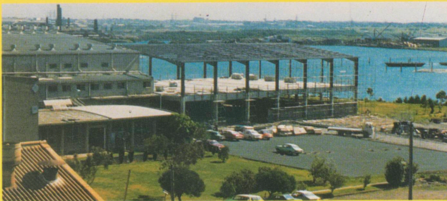
These extensions to Union Carbide's polyethylene plant are being built under Fletcher's guaranteed price scheme. The requirement of high loading (450lbs per sq. ft) on a suspended concrete floor was the main design consideration.
