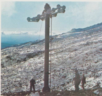
BELOW: High in the thin cold air, workmen secure the crossbar section ("yoke") to one of the pylons.
