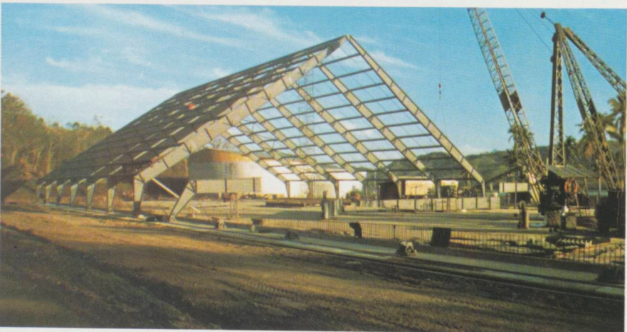
LEFT: Two major construction jobs in Fiji in which Fletcher Construction is closely involved are (above) Fiji's first multi-storey carpark and (below) extensions to the Fiji Corporation's facilities at its sugar mill near Labasa. Shown under construction is the bulk sugar store, which will have a capacity of 30,000 tonnes.
