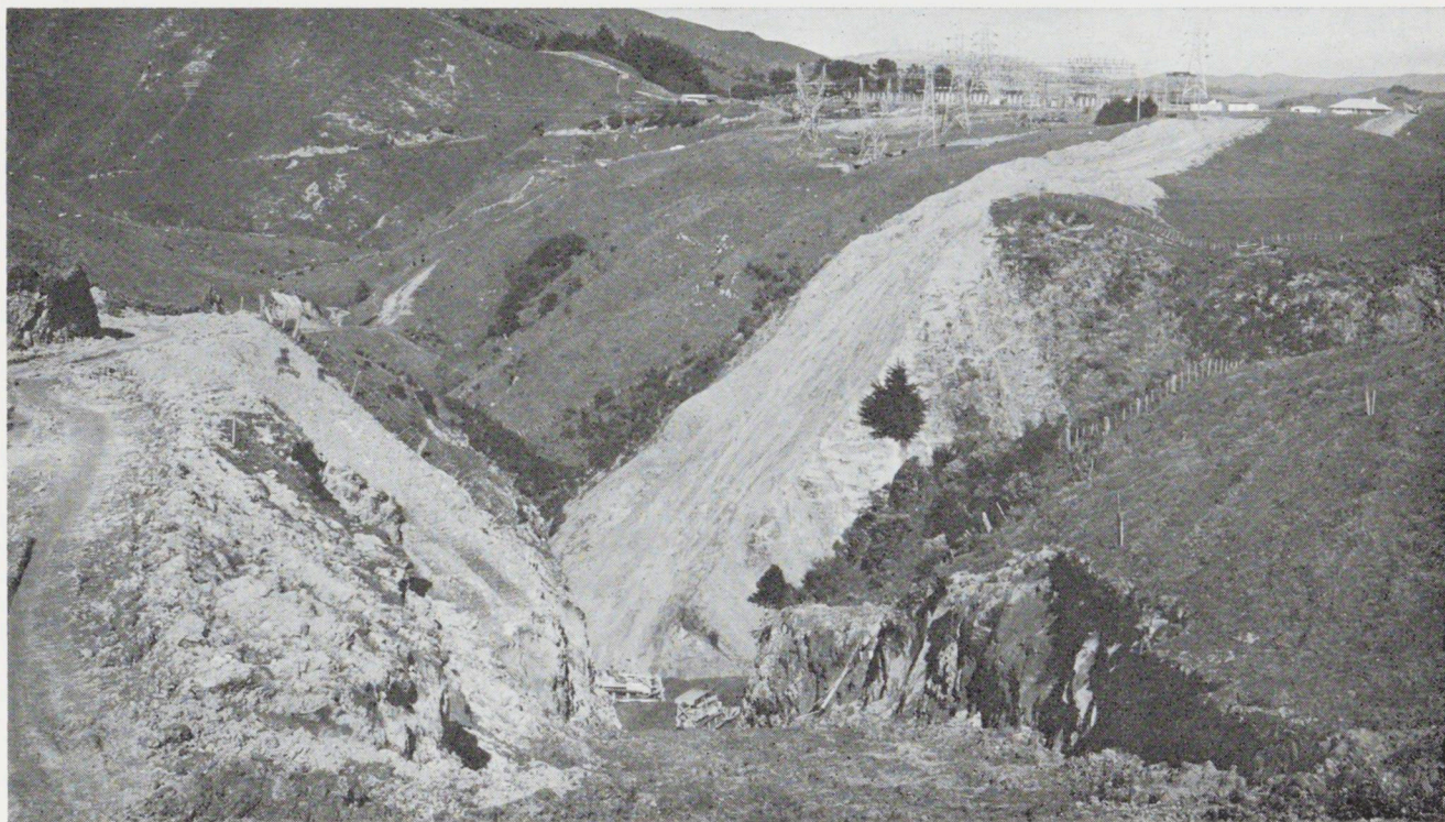
A steep stretch of country on the Tawa - Plimmerton section of the pipeline which was the first to be started.
