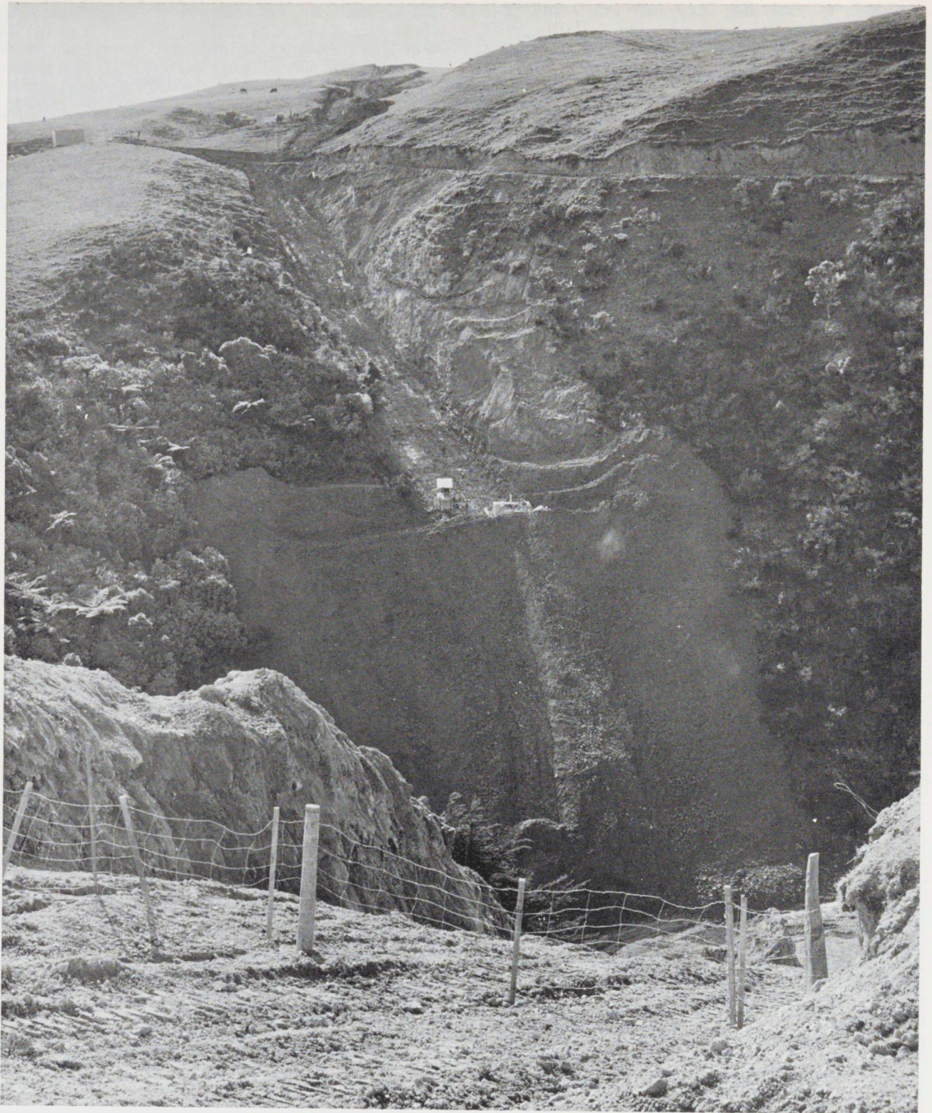
Another view of the rugged country being worked near Porirua. The pipeline route is indicated by the earthworks in the centre of the photograph. The fence in the foreground is a temporary one erected to contain stock when the permanent fence was taken down to allow the work to be carried out.
