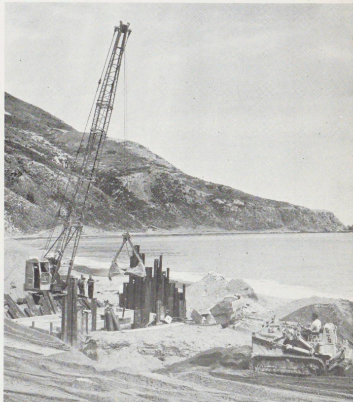
Building the joint pit at Oteranga Bay — one of the jobs in Fletcher Construction's sub-contract.
