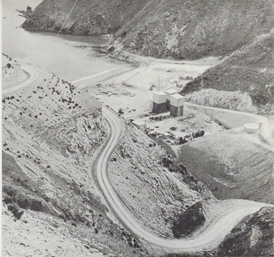
Fighting Bay (north-east of Blenheim), the South Island terminal of the Cook Strait cable.
