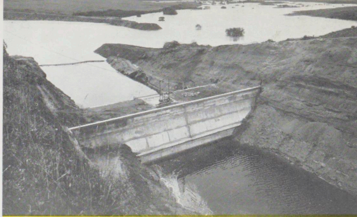
Control gate structure at entrance to canal.
