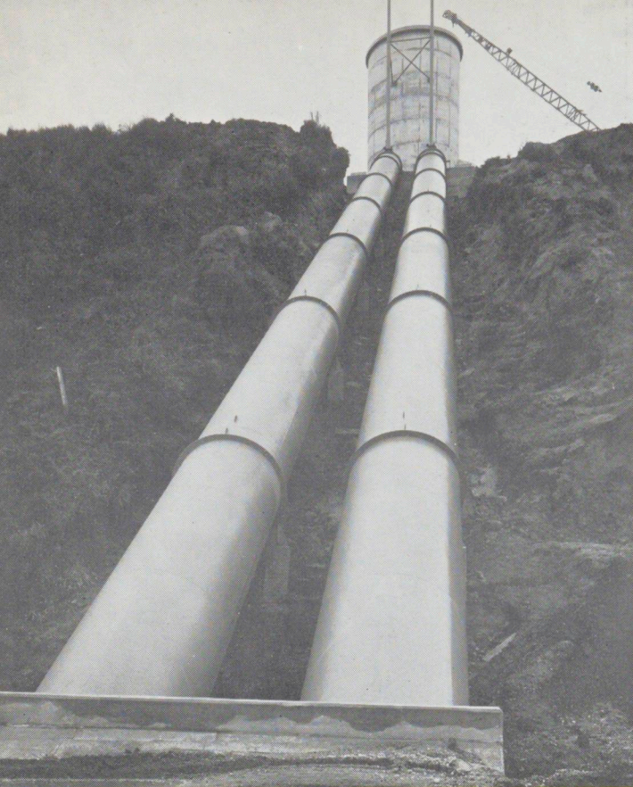
LEFT: A general view of the project with the lake forming, water in the canal and power house under trial.
